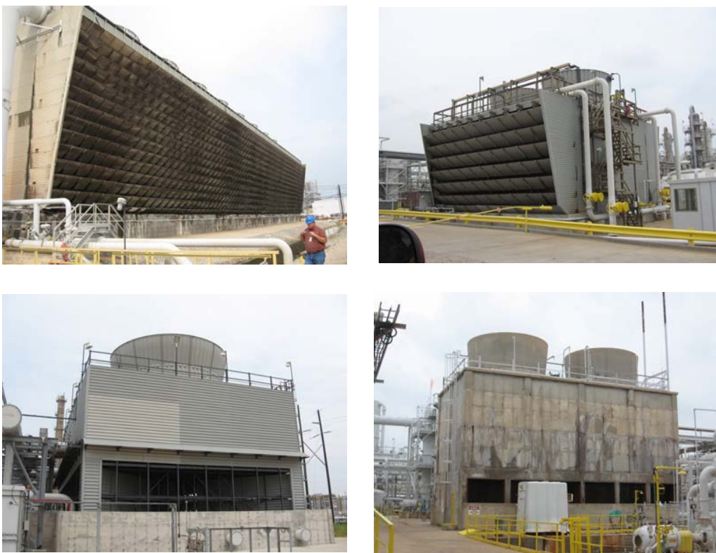
Figure 92. Examples of Cooling Towers (Top Left: 9-Cell Wooden Tower; Top Right: 2-Cell Wooden Tower; Bottom Left: 2-Cell Concrete Tower; Bottom Right: 2-Cell Fiber-Reinforced Plastic Tower)
