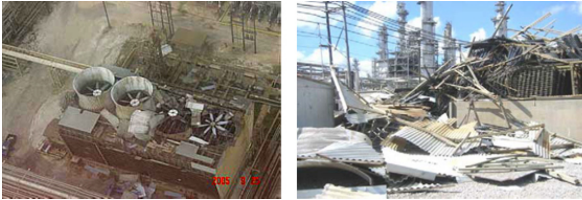
Figure 93. Observed Hurricane Damage to Cooling Towers
