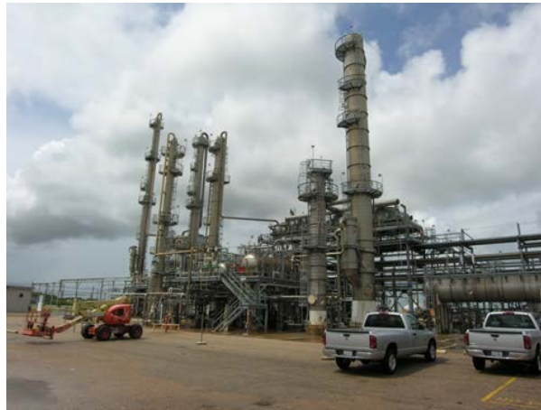
Figure 94. Example of a Process Tower
