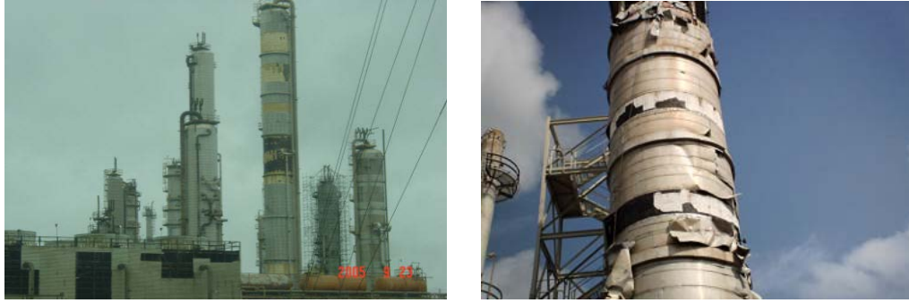
Figure 95. Observed Hurricane Damage to Process Towers
