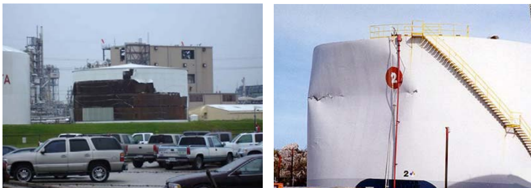
Figure 88. Observed Wind Damage to Storage Tanks
